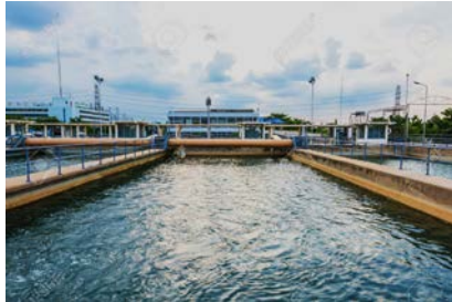
WATER TREATMENT (WTP)
