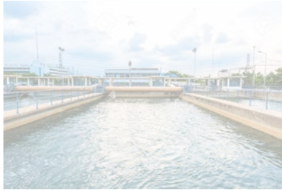
WATER TREATMENT (WTP)
